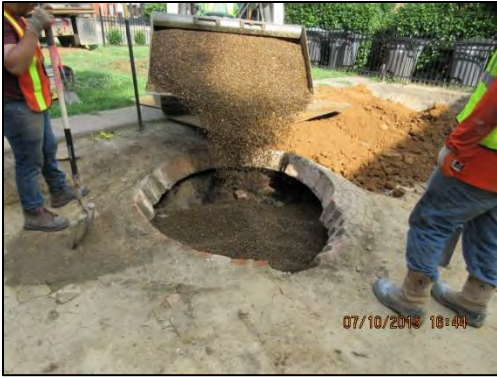
One of the cisterns uncovered during soil removal at the Jacobsville Site being capped with pea gravel, Evansville, Indiana
