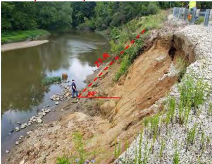
Active streambank failure along the Vermilion River (Vermilion County, Illinois)
