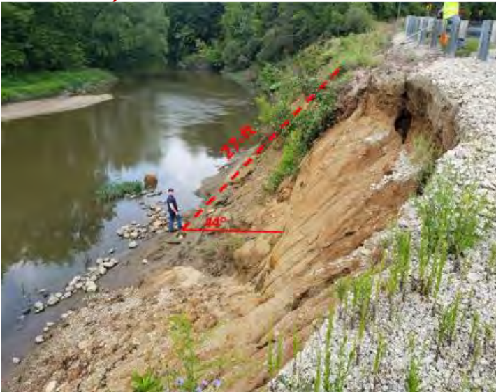
Active streambank failure along the Middle Fork Vermilion River (Vermilion County, IL)
