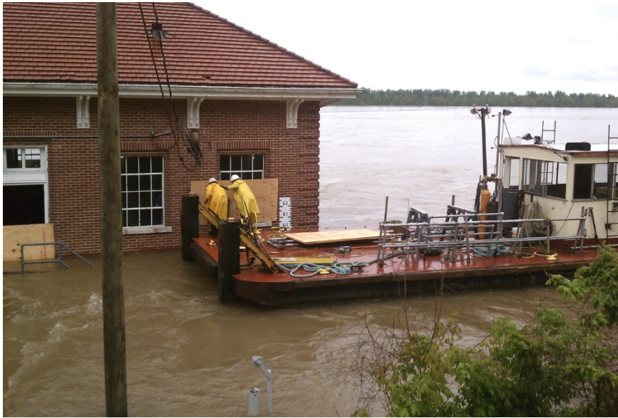
Figure 16: The crew at Lock and Dam 53 on the Ohio River Covers the power house windows with plywood to keep drift from breaking them as the river rises in April 2011.
