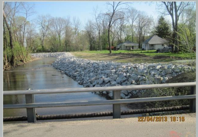
Photos are of the Feather Creek Project in Clinton, Indiana. Top photo shows project in action before it was even completed.
